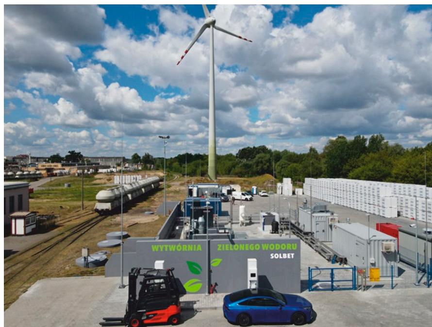
Figure 7. Green hydrogen production plant in Solec Kujawski [51].
