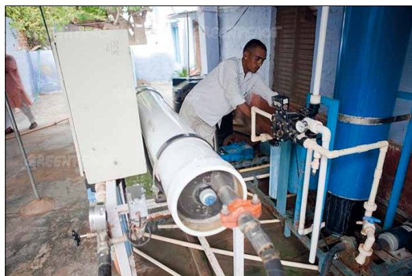
Rys. 14. Solar-powered Reverse Osmosis Plant (fot. Prashanth Vishwanathan, Greenpeace)
