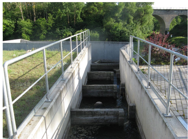
Fig. 7 The fish ladder at a small hydropower plant Wierzycza (Pomorskie Voivodeship) (photography: B. Igliński)
