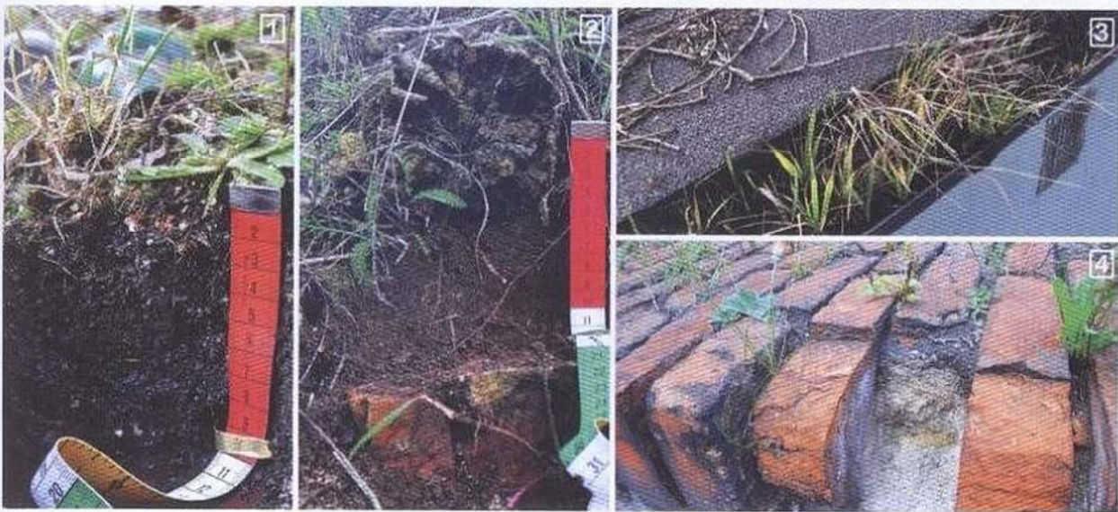
Fig. 5.3-4. Examples of soils forming on buildings: 1 – Isolatic Technosol (Arenic, Humic); 2 – Isolatic Technosol (Loamic, Humic); 3 – Isolatic Technosol (Folic); 4 – Isolatic Technosol (Arenic).
