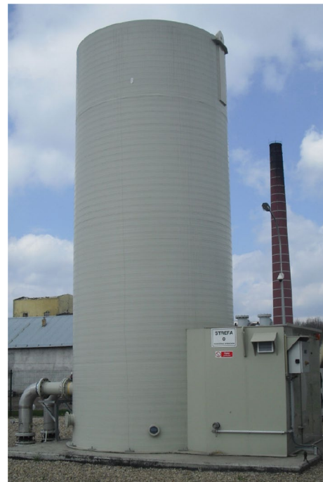
Fig. 9 Biogas desulfurizer in the biogas plant in Liszkowo (photograph B. Igliński)
