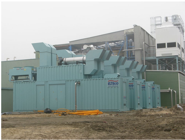
Fig. 8 Cogeneration systems in Melno (photograph B. Igliński)
