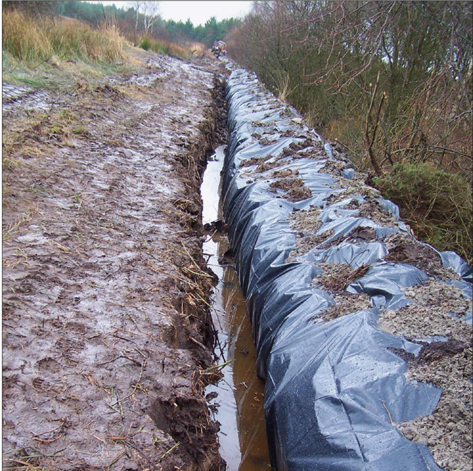
Figure 5. Installment of screens (PCV foil) to seal the edges of the peat-bog dome (photo by Magdalena Dąbkowska)
